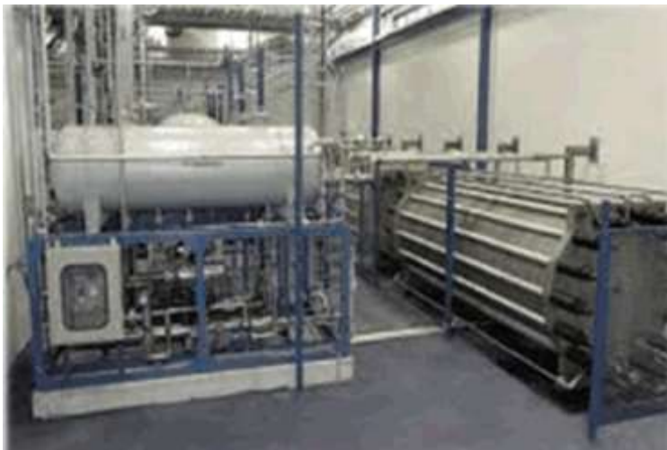
Middle-size Electrolysis (10-20MW)
