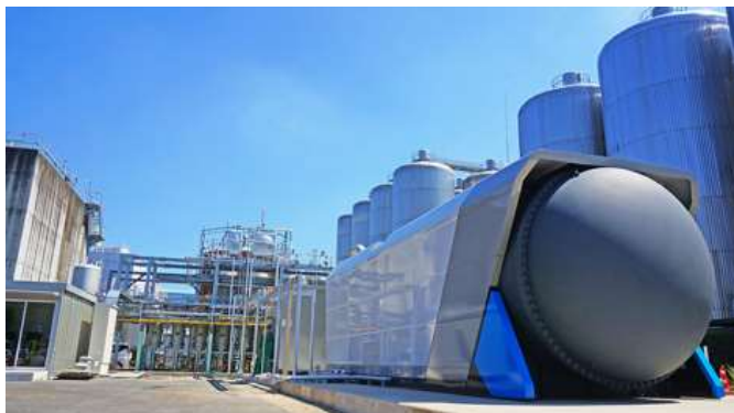
Biogas SOFC at Asahi Breweries Ibaraki Brewery
